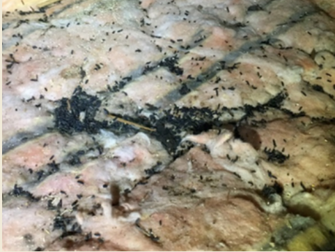
Guano laying on insulation of attic floor.
