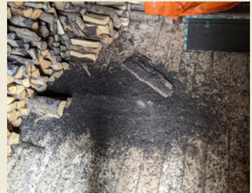
Guano laying on ground below the ridge line of an old granary where a large maternity colony roosted.
