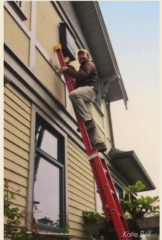
Installation of a four-chambered bat house on the side of the building prior to sealing the roost.
