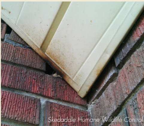
A gap between the wall and the soffits, along the roof edge, used by bats to access the attic. There is brownish staining from the oils of the bat's fur repeatedly rubbing off onto the surface during entry.
