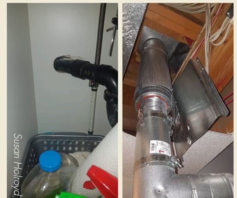
Check under sinks and in basements where plumbing or HVAC passes through walls or ceilings. These points may provide bats access to inside your home.
