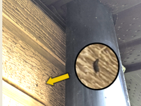
Guano stuck to siding of exterior wall near rain spout.
