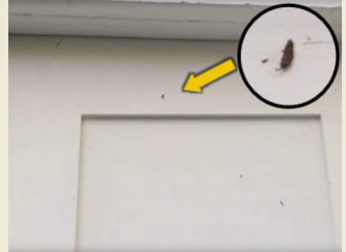
Guano stuck to the exterior surface of a door.
