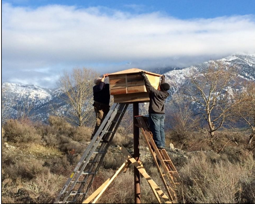
Figure 14. A mini condo is installed in late fall at Lillooet, British Columbia. Photo contributed by V. Birch-Jones. This structure is larger and offers more roost microclimate options than a standard multichambered bat box. This particular design was modified to contain a pillar of sand in the middle to function as a heat sink – stable and warm at night for pups, but unlikely to overheat despite the fact that this region is typically the hottest location in Canada (outdoor ambient temperatures have reached 47°C or 117°F; Environment Canada 2021). This site will continue to be monitored for effectiveness.
